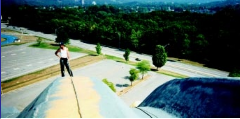
The University of West Virginia chose SPF for the 174,000 sq. ft. roof of the Evansdale Coliseum (above, cover). The SPF roof was installed in 1975 and recoated in 1991.
