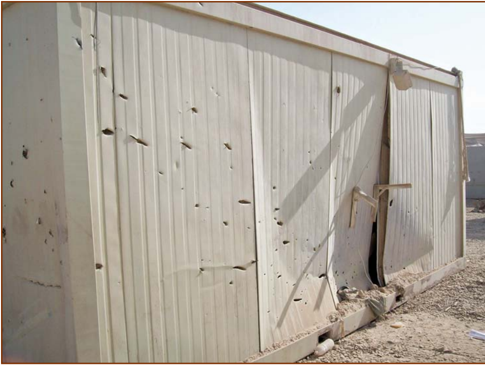
Figure 18 – This metal building was approximately 50 yards from the mortar shell's impact.
